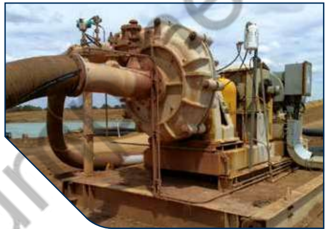
After installing AESSEAL® double seal and tank system
