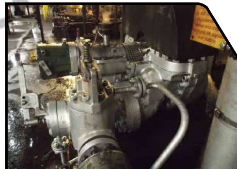
With Steam Turbine Seal
