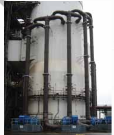
Power Station Absorber
