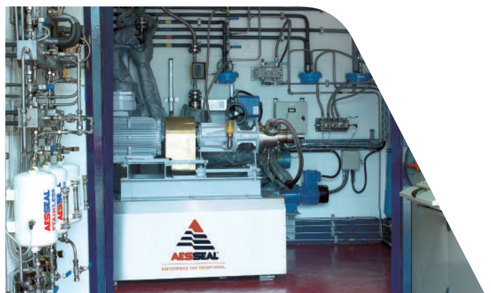
Extensive AESSEAL® test facilities
